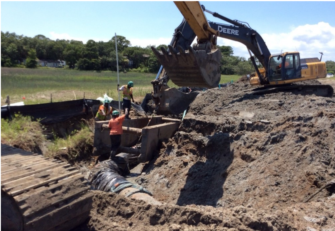
A crew works on the relocation of the PSD’s 24-inch water transmission pipeline in greater Bluffton.
