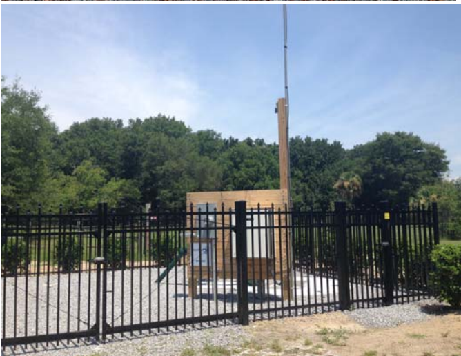
The PSD's new Mid-Spanish Wells, top, and Baygall sewer pump stations.
