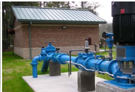
Upper Floridan Well & Pump
