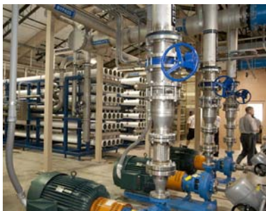
Interior of the RO Facility
