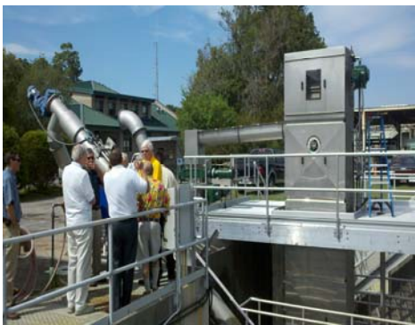
Wastewater treatment headworks
