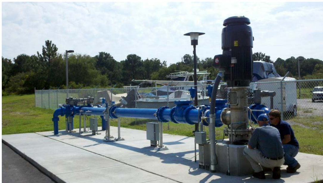
In 2011, the PSD completed construction of its Aquifer Storage & Recovery Well in Hilton Head Plantation. The well stores water in the underground aquifer in the winter months of lower demand, and withdraws water in the summer months of high demand – providing 2 million gallons a day over an approximately four-month period.
