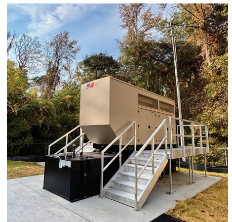
Generator for the new Booster Pumping Station
