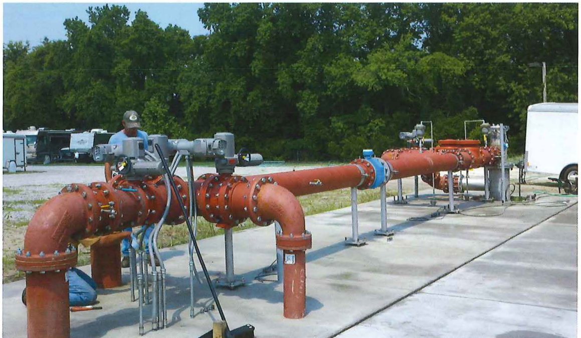
Hilton Head PSD's new Aquifer Storage & Recovery (ASR) well is located off Royal James Drive in Hilton Head Plantation. The well stores treated drinking water during the winter months of low demand and withdraws it for re-treatment and distribution during the summer months of high demand. This is Hilton Head Island's first-ever ASR well. It is needed in order to ensure a long-term and high-quality supply of drinking water in the face of ongoing saltwater intrusion into the island's traditional groundwater source.
