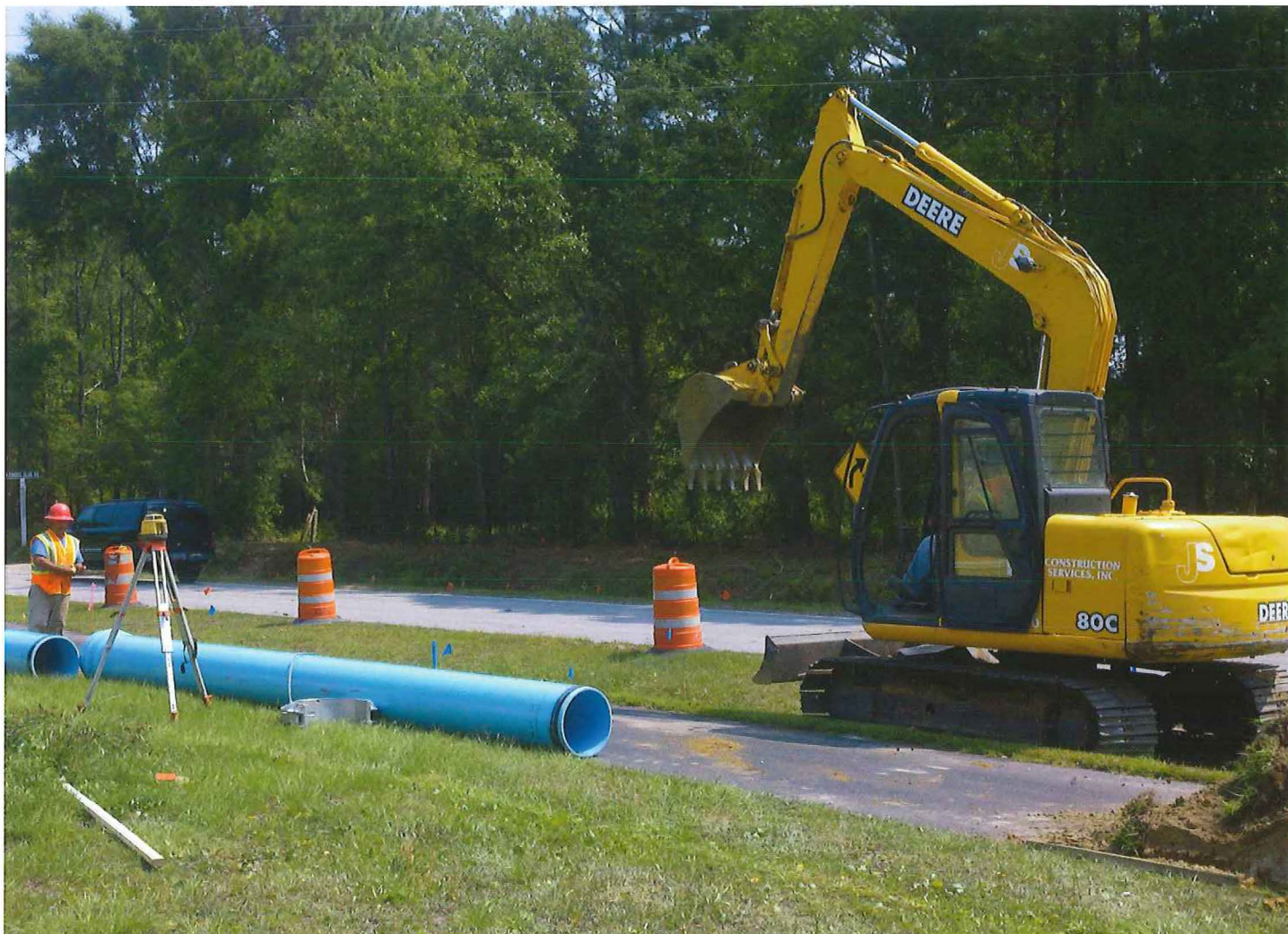
The PSD is installing a water transmission main in the Wildhorse and Gumtree roads area as part of a water supply project to combat the effects of saltwater intrusion in our traditional groundwater source.
