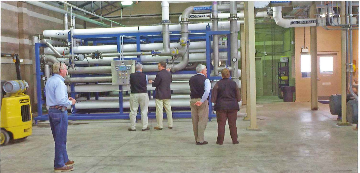
Edisto Beach officials toured the PSD's Reverse Osmosis (RO) Plant recently to learn about the process as they consider constructing a smaller plant for their community. Edisto Beach, like Hilton Head Island, is faced with lost drinking water supply as a result of saltwater intrusion into their groundwater source. The PSD's RO Plant is a key tool in the fight to replace supply lost to saltwater intrusion.
