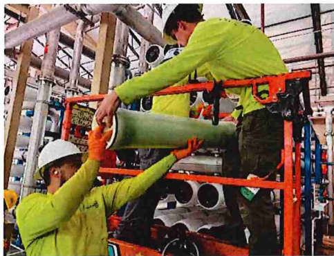
Loading membranes into the new RO filter skids
