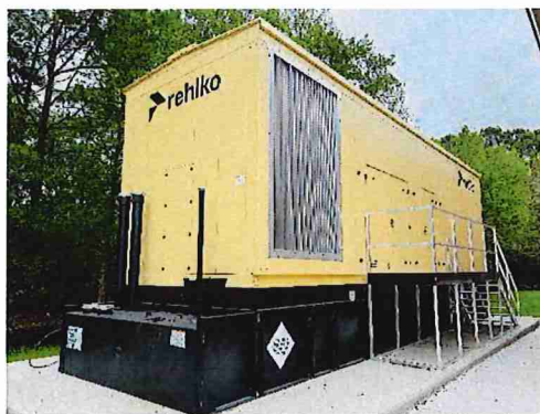
RO Plant Emergency Generator
