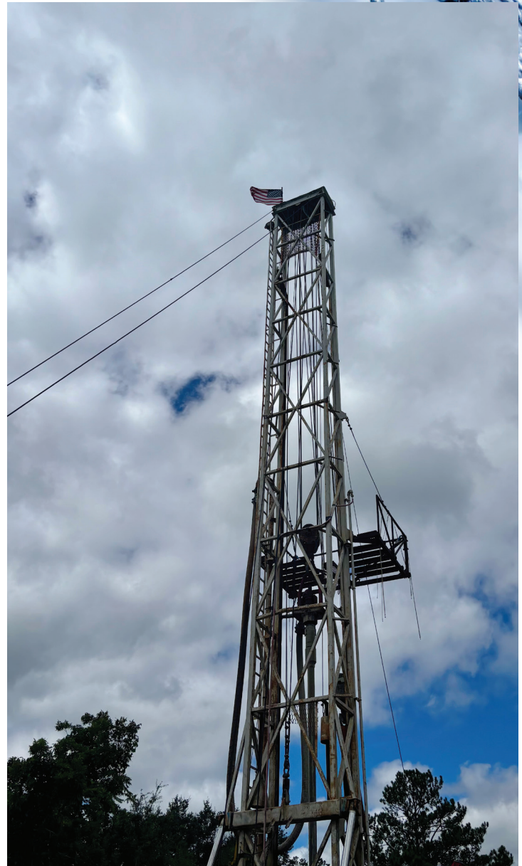
The drill rig for the deep well at the Old Welcome Center location
