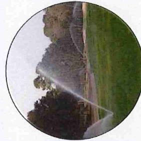
Recycled Water Distribution
