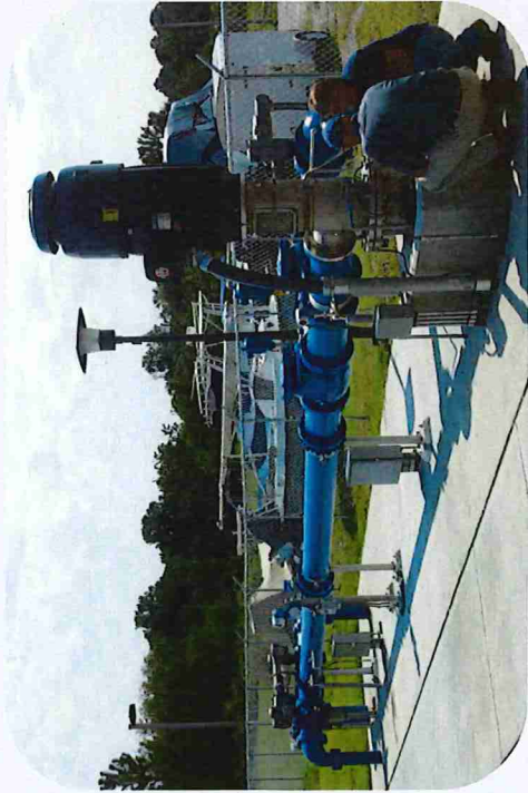
HHPSD's ASR Facility at Royal James UNESCO Managed Aquifer Recharge Worldwide Example
