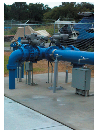
The PSD’s current Aquifer Storage & Recovery Well facility. The PSD is working to construct a second ASR Well.
