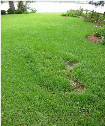
Failing septic system on north end of Hilton Head Island with Intracoastal Waterway in background.
