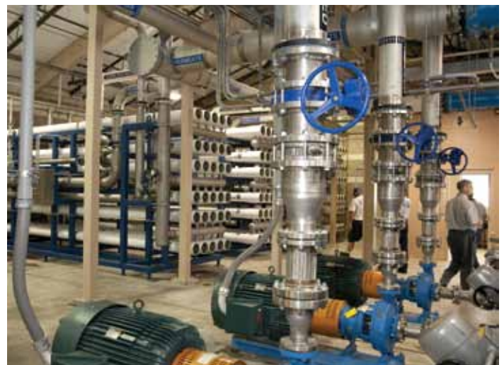
The interior of the PSD's Reverse Osmosis (RO) Plant. The plant currently provides about 40 percent of our water supply and is being expanded to provide even more water.
